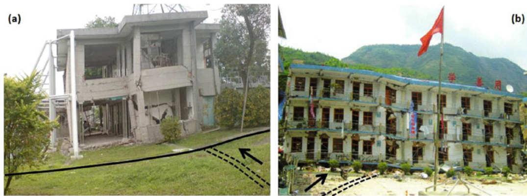
Fig. 1 Examples of structural damage due to reverse faulting: (a) severe damage of a 2-story building subjected to a fault offset of about 1.5 m during the 1999 Chi-Chi earthquake; (b) partial collapse of a 3-story building, subjected to a fault offset of about 1 m during the 2008 Wenchuan earthquake in China (adapted from Lin et al. , 2009)
