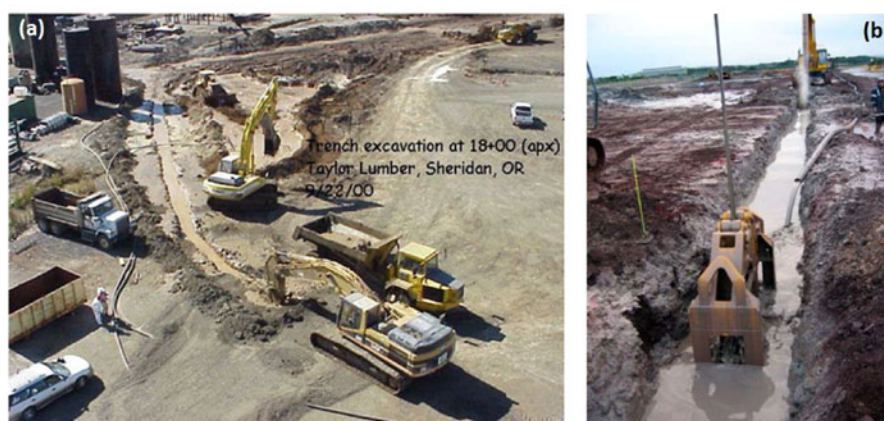
Fig. 2 Soil bentonite wall (SBW) under construction: (a) distant view; and (b) close view (adapted from McKnight et al. , 2001)
